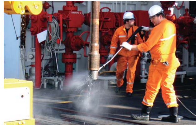
A roughneck (engineer) washing the joined portion of the pipe. The machine conducts most of the heavy works and the roughneck supports these operations.
