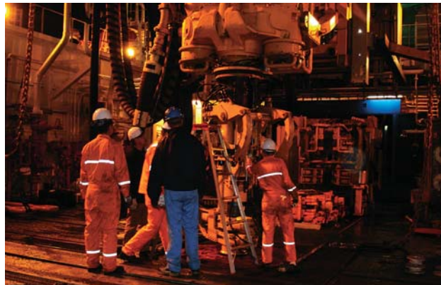
Operations continue after sunset. During test operations, operations were conducted on a 12-hour basis. During actual operation, drilling operations will be conducted on a 24-hour basis.
