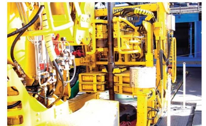
Hydraulic Roughneck (the machine in the background of the Photo) for tightening the threaded ends of the pipes to connect and loosening the threaded ends to disconnect.
